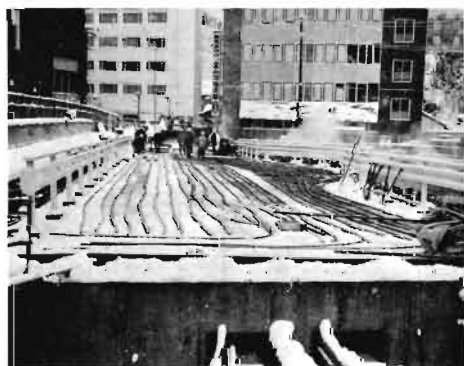
図30 ヒートパイプ布設状況 Construction site of corrugated long heat pipes on bridge
